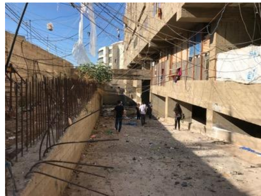
Fig. 26. Electric wires in Ouzai shelter
